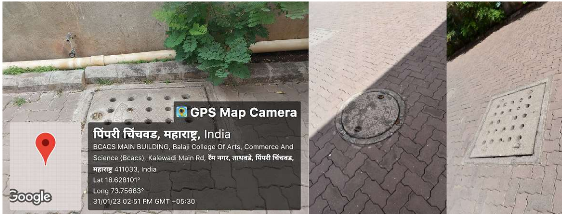
Liquid Waste Management Chambers at BCACS
